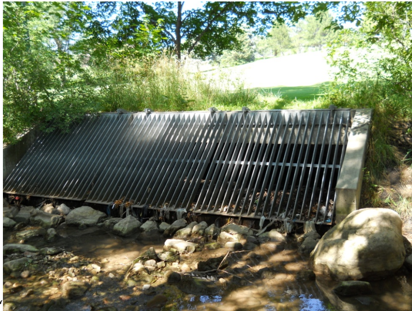
Photo 32: Parleys Creek below 1700 E, large outfall along north (secondary) channel, approximately 100-150 ft. downstream of 1700 E culvert outlet.
